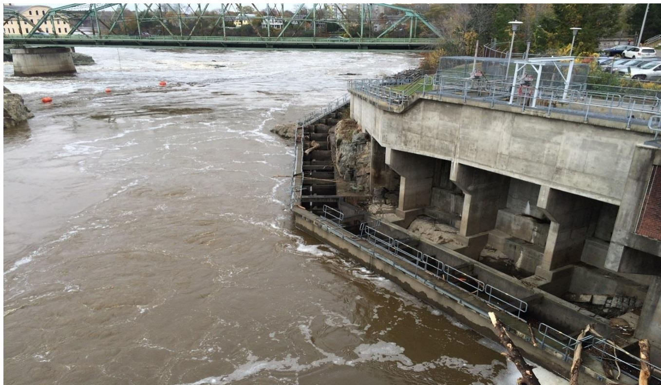
Figure 4. Damage to lower fishway railings during high river flows in October resulting in the closure of the fishway on October 30, 2017
